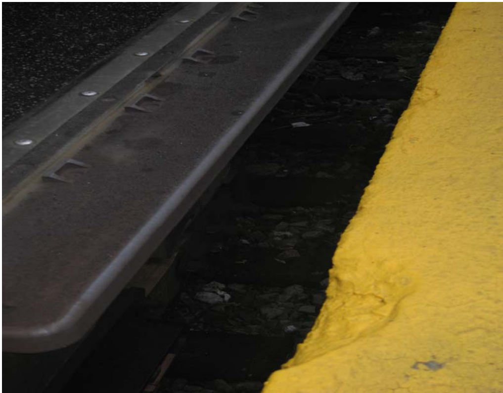
Holes in the platform at the entrance of the subway door at the Avenue M Station of the Q line.
