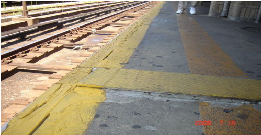
Corrosion throughout platform at the 4 th Avenue Station of the F line.
